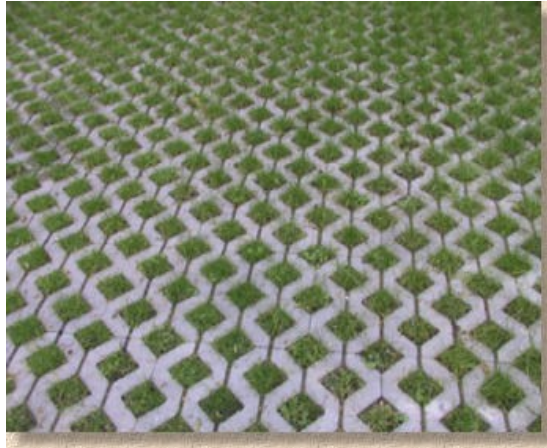
Modular concrete pavers that fit together with funnel-like openings installed over an infiltration storage bed of uniformly graded limestone (below)
