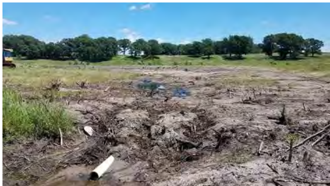
Photo 1: Tree removal and tile breaks
